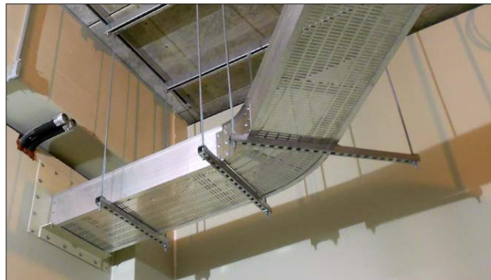
IMMEDIATE RIGHT—Installed AB-COPE Cable Bus system featuring a firestop/wall seal.
