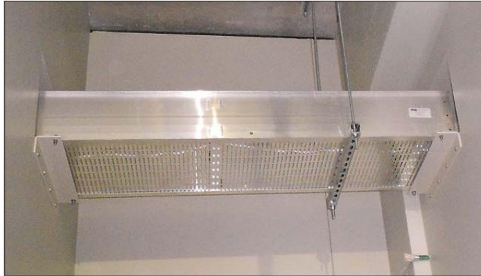
IMMEDIATE LEFT—Installed AB-COPE Cable Bus system featuring two sequential wall penetrations/seals with firestops .
