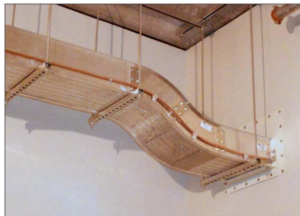
ABOVE—Cable Bus system with external grounding cable and firestop/wall seal.
