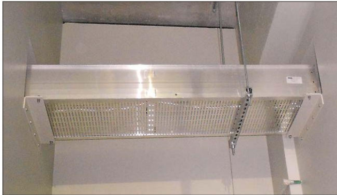
IMMEDIATE LEFT—Installed AB-COPE Cable Bus system featuring two sequential wall penetrations/seals with firestops . LOWER LEFT—Installed Advanced Cable Bus system (in a trench) featuring a wall penetration/seal .
