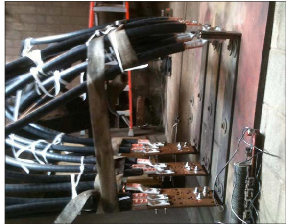
ABOVE—A short-circuit test being run on an Abcope Cable Bus system.
